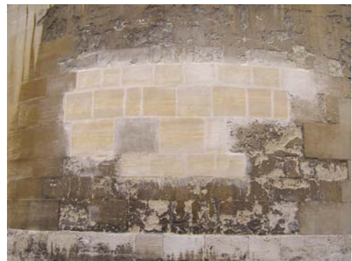
Fig. 8. Replacement of a section of wall in Oxford previously destroyed by catastrophic decay of Jurassic oolitic limestone (approximate image width 6 m).
