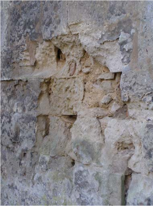
Fig. 4. Catastrophic decay of a section of wall constructed of Jurassic oolitic limestone, Oxford (approximate image width 4 m).
