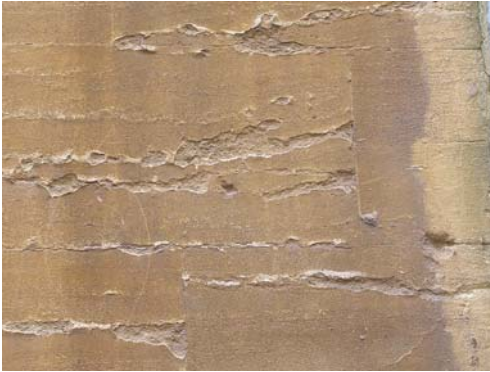
Fig. 5. Decay of a Jurassic oolitic limestone initiated along clay partings within the stone, Oxford (approximate image width 1 m).
